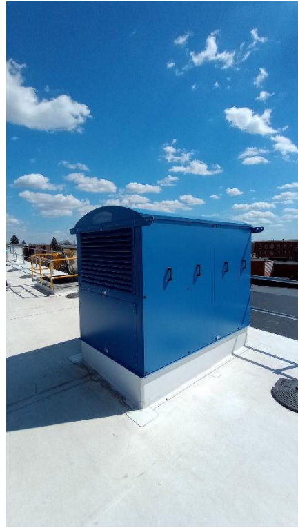
Rooftop energy recovery unit.
