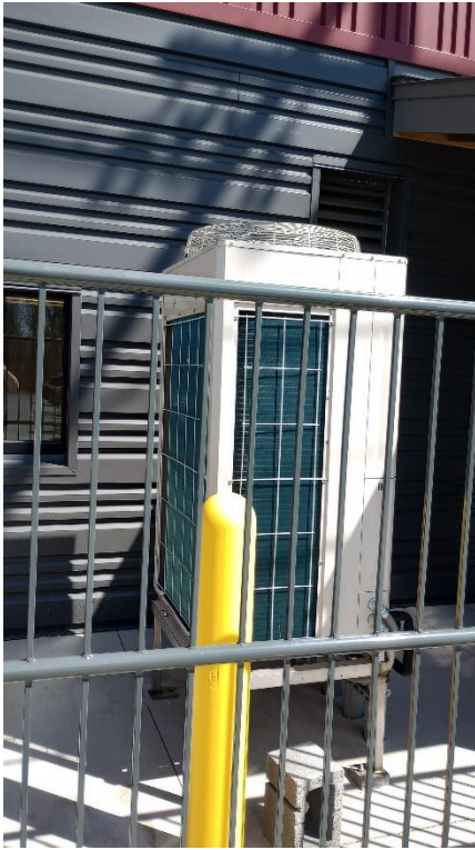
Outdoor VRF unit.
